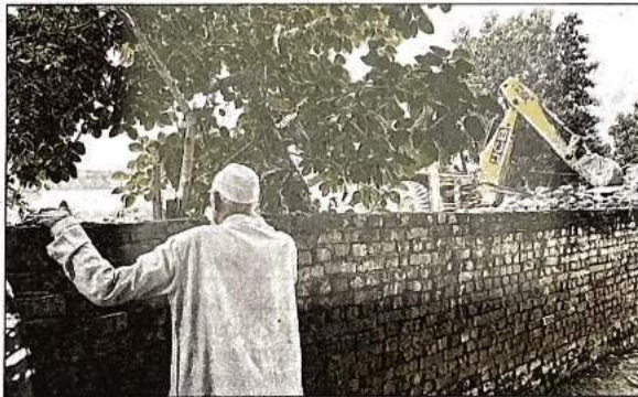
Residents said the demolition started at 10am and was over in an hour
