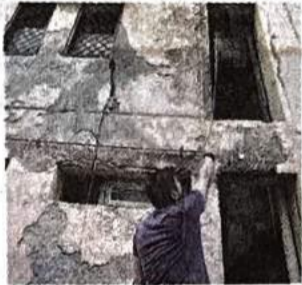
A resident pointing at a damaged portion of the housing complex. FILE PHOTO
