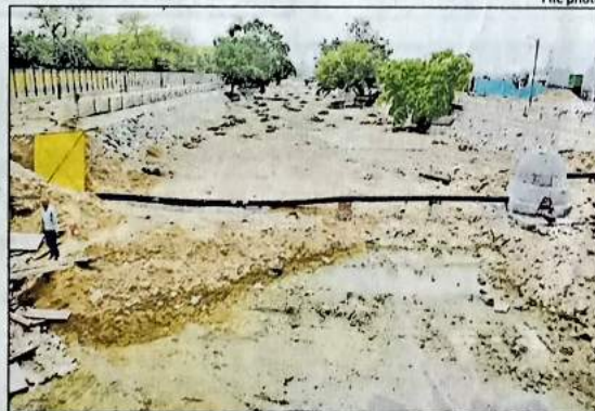
A DDA official said the drain was being constructed along the boundary wall of the airport opposite Sector 8 and would be linked to the upstream and downstream sides of trunk drain 2
