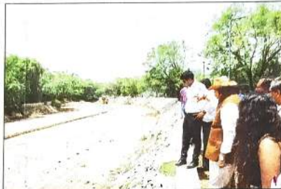
The LG secretariat said the drain was almost 95% built and likely to be ready by next month
