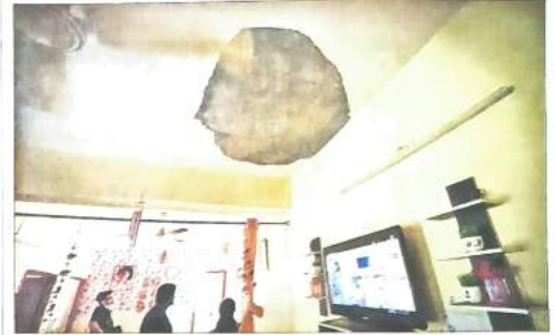
The portion of the ceiling that fell in the drawing room.
