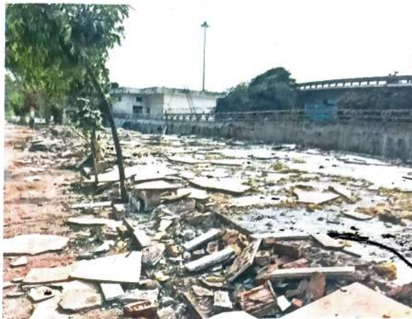
The demolition took place close to the Yamuna near Kashmere Gate ISBT. Express
