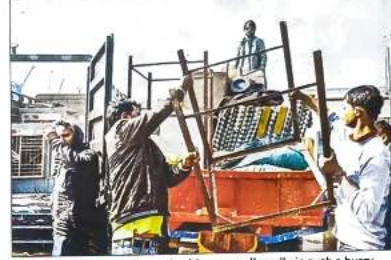
LEFT IN THE LURCH: The authorities were allegedly in such a hurry that even salvageable items such as a water tank and grilles, which could have been reused elsewhere, were razed
