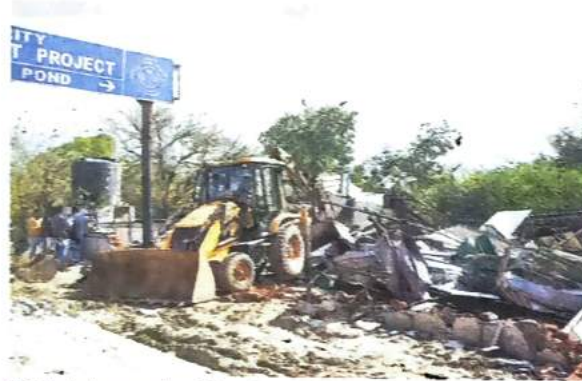
Night shelter number 235 at Sarai Kale Khan being razed during a demolition drive on Wednesday. SHIV KUMAR PUSHPAKAR
