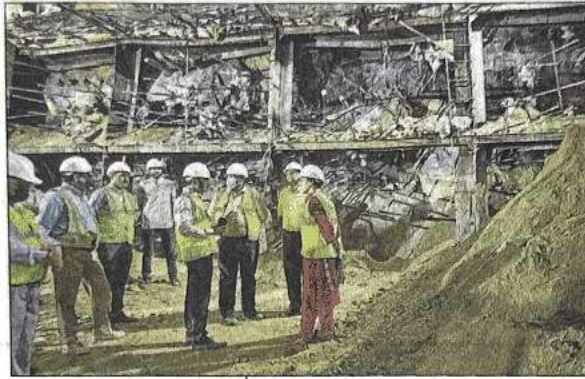
PWD minister Atishi inspects the Bhairon Marg underpass, part of the Pragati Maidan tunnel project, on Thursday. HT PHOTO
