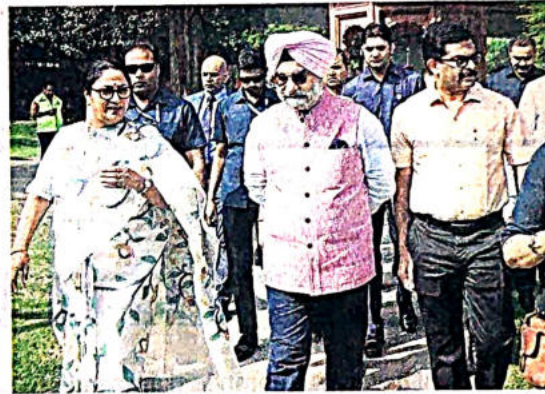
CM Rekha Gupta and L-G Taranjit Singh Sandhu inspecting ongoing works at Vasudev Ghat on Wednesday. SHIV KUMAR PUSHPAKAR
